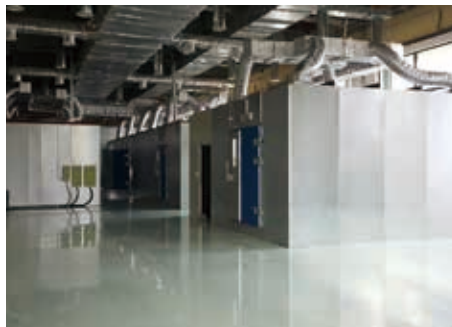
RF Shielded Room
